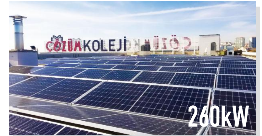
Project Type: Commercial Rooftop Location: Turkey / Ankara Commission Date: 2021-11 Product: SRP-450-BMA-HV
